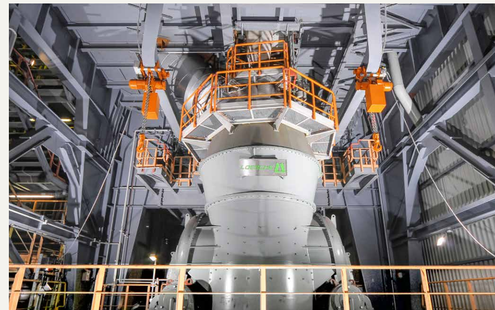
Cement mills incorporating vertical mill drives
