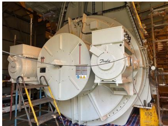
Figure 62: IFPS® with two generators mounted on a two stroke diesel engine
