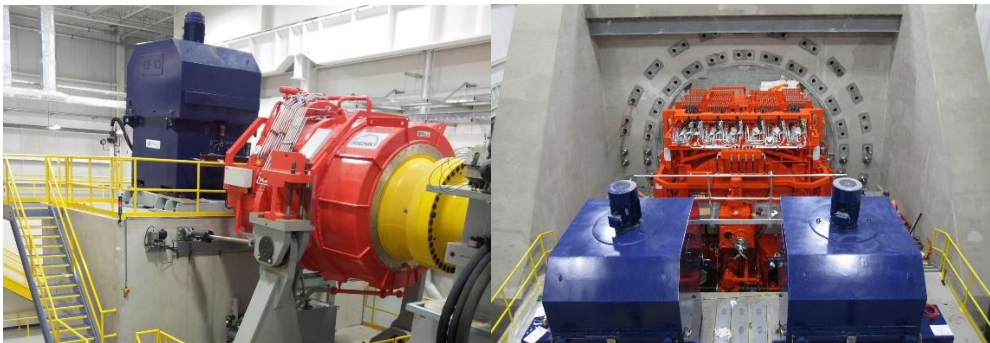
Figure 61: Motor-Gearbox-Drive-System for a 7.5 MW (left) and 15 MW (right) Wind Power Nacelle Test Rig
